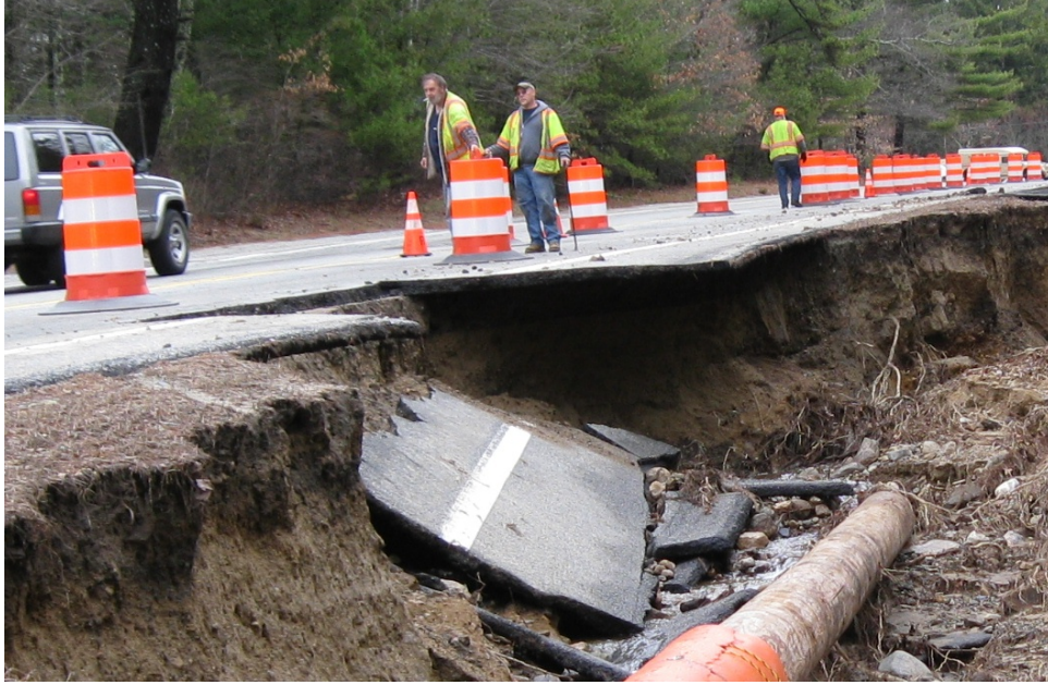
Undercut road way, Route 165. Photo courtesy of Sheila Reynolds-Boothroyd.
